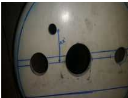
Figure 5.2. Orifice Retrofit. Orifices in a pipe cap that controlled water flowing into the dry well at the Corporation Yard. Knowledge of the flow rate each orifice permitted with a given head supported the calculation of infiltration volume.
