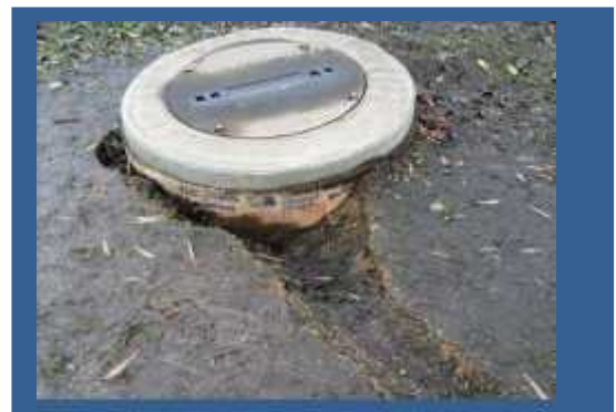
Dry Well - Erosion
