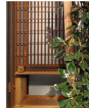
Example of Metal Grid Panel (Overall)
