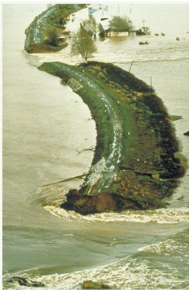
Figure 4-85 1986 Tyler Island Levee Breach
