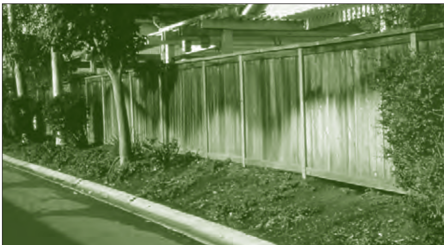
Damage to fencing from sprinkler irrigation.
