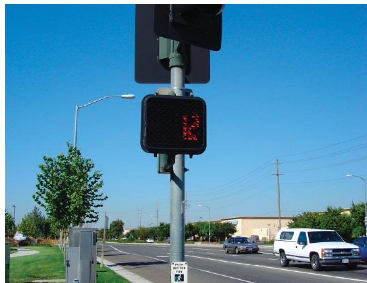
New countdown crosswalk signals let pedestrians know how much time remains for them to cross the street.
