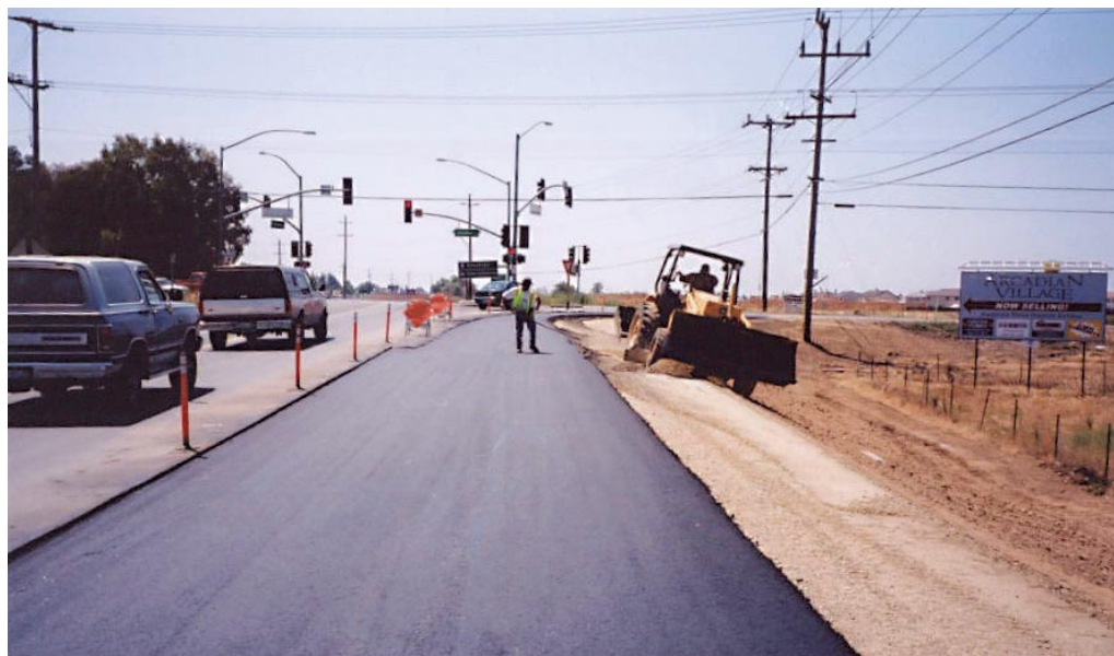
Road crews repave and widen the southbound West Stockton Boulevard exit from Highway 99 to Sheldon Road.
