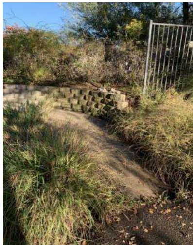
Figure 30. Overgrown foliage obstructing ramp access by northeast trailhead off Bond.
