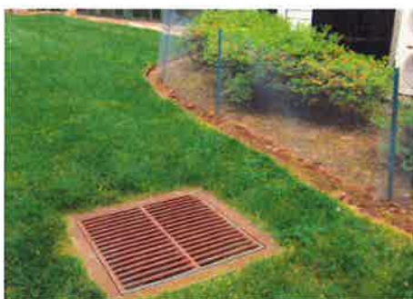
Figure 2. Dry well installed to receive runoff flowing through a lawn (Source: R. Pitt)
