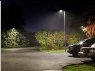
Parking lot lighting
