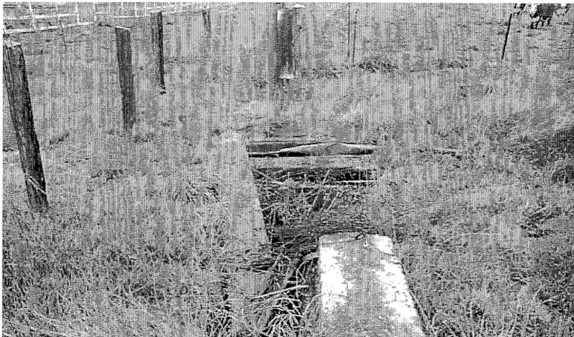
Pictured above is a timbers and debris covering the underground concrete vault box with gutter observed within the Property and at the approximate mid-point of the western boundary of the Property. Pictured in the background is a power pole that brings power lines to the Property servicing the agriculture water well.
