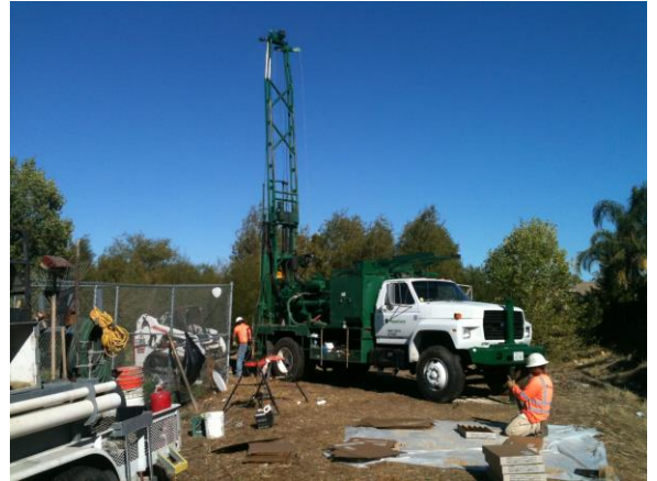
Exhibit 7. Site 1: Residential Site - Strawberry Creek Water Quality Basin Drilling of Investigation Borings/Monitoring Wells
