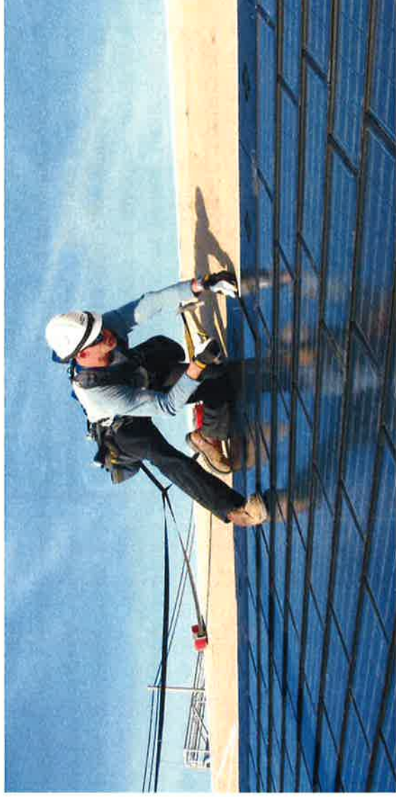
Integrated solar roof panels
