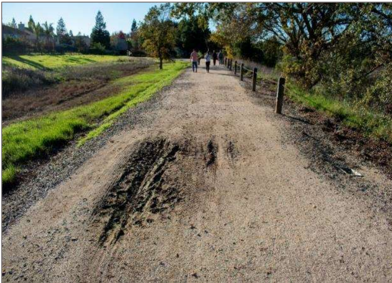
Figure 15. Ruts due to erosion on unpaved portion of trail.
